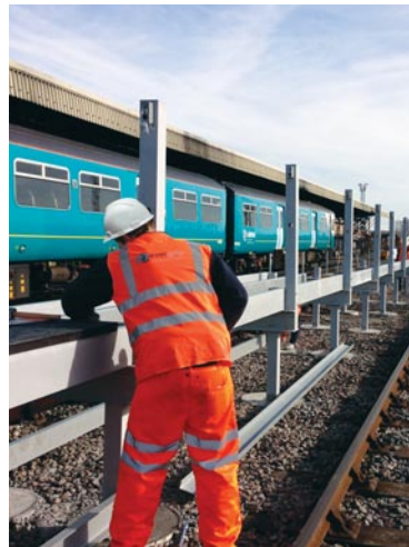
Access Platforms & Ramps
