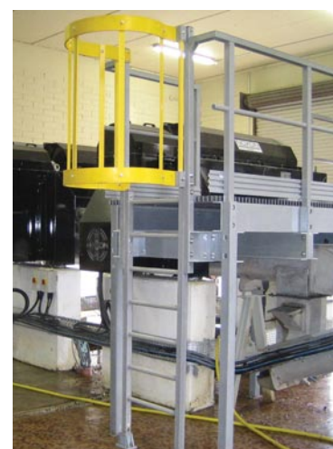
Fixed Access Ladders
